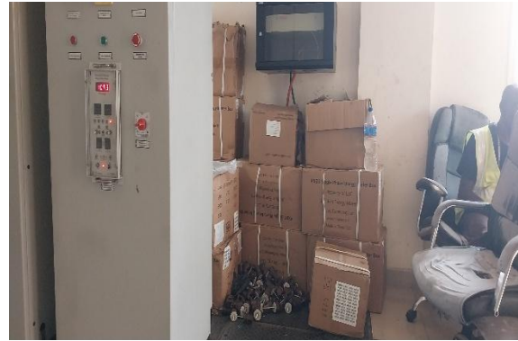
Materials Store Behind Switchgear/Kle Sub.
