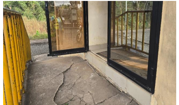
Entrance of the Kle Substation
