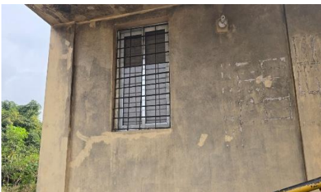
Damaged Window Bar at Kle Sub.
