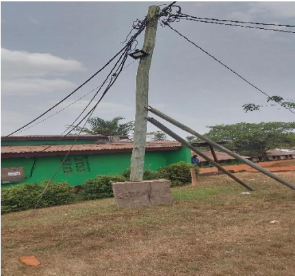
Leaning LV Pole Supported with Metal/KRTTI
