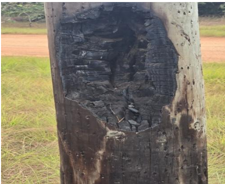
Burned MV Pole along Robertsport
