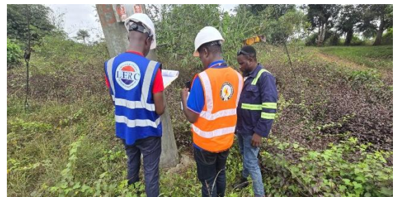
Failed/Sinking 66kV Foundation
